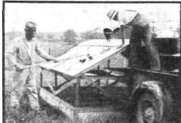
Range shelters covered with insulation board should be given a thorough coating of liquid asphalt roofing. It can be applied with a brush.
