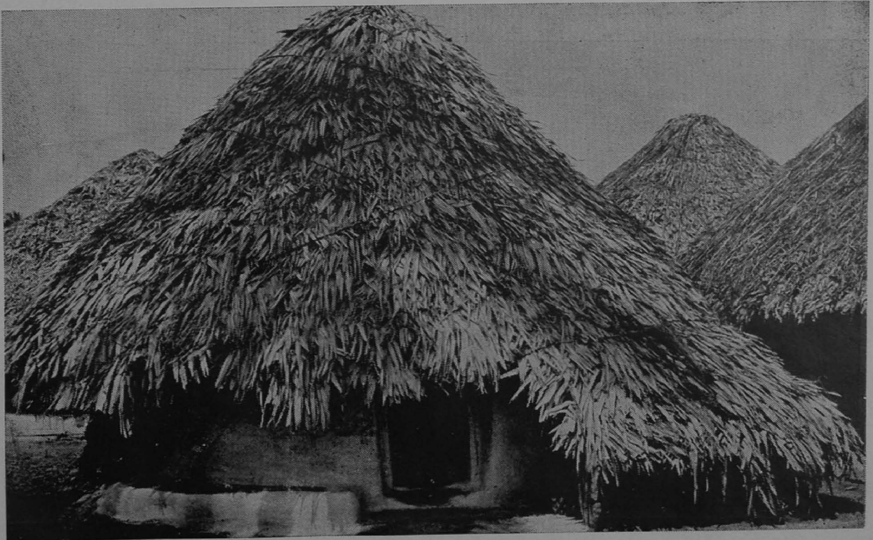
For thatching, palmyra leaves which are available in plenty in the village are used and these would last for three to four years only. Because of the unworkable size of the Palmyra leaves, the roof would present an irregular appearance.
